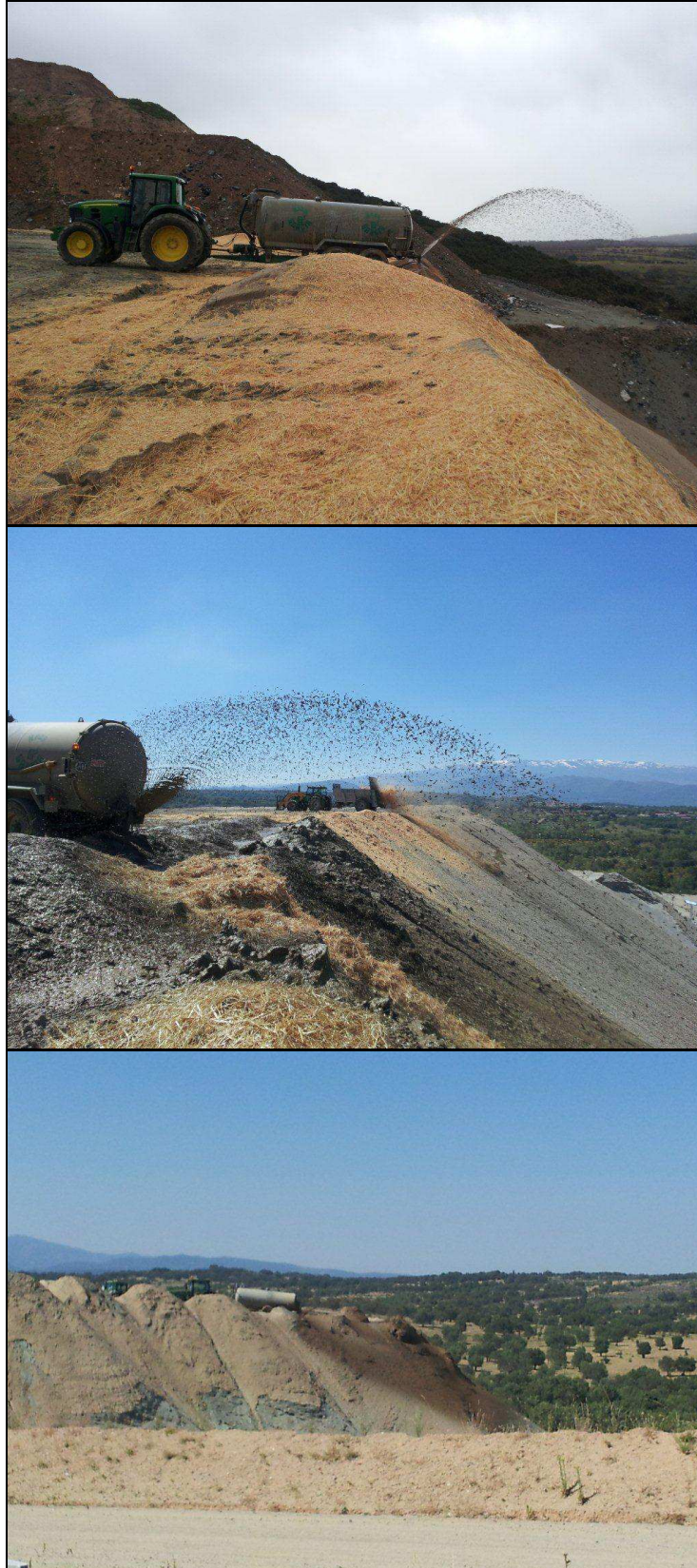
Figure 17-3. Dust Control System
